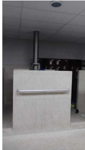
GIRLS LOCKER ROOM - DEMO (E) TERRAZZO WALLS, SHOWERS AND ACESORIES
