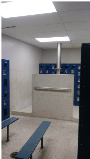
BOYS LOCKER ROOM - REMOVE & SALVAGE (E) LOCKERS, DEMO BENCHES, TERRAZZO WALLS, SHOWERS & ACCESSORIES
